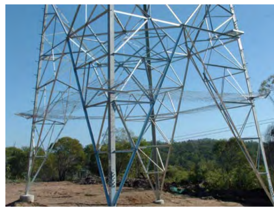
Fauna friendly anti-climbing barrier installed on transmission structure
