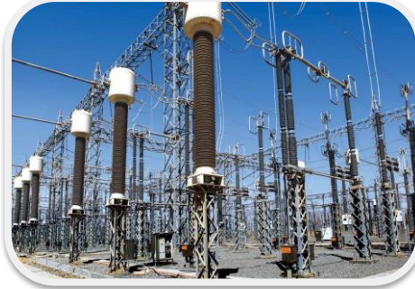
2923 km power transmission line with 1000 km HVDC
