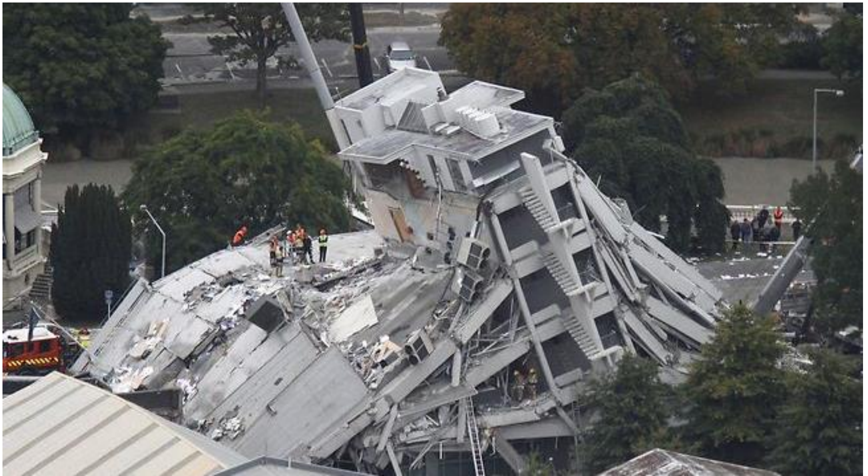
The PGG building after the February 2011 earthquake. The Avon River is in the background.
