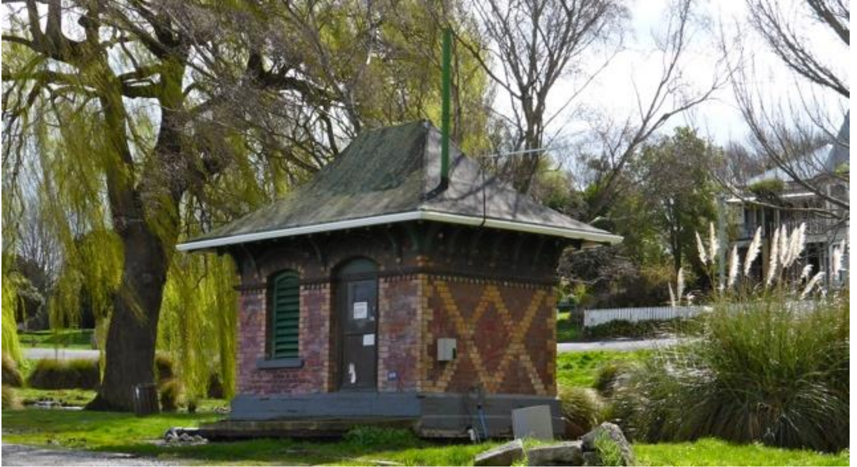
One of the pump stations on the Avon River. Note earthquake damage.
