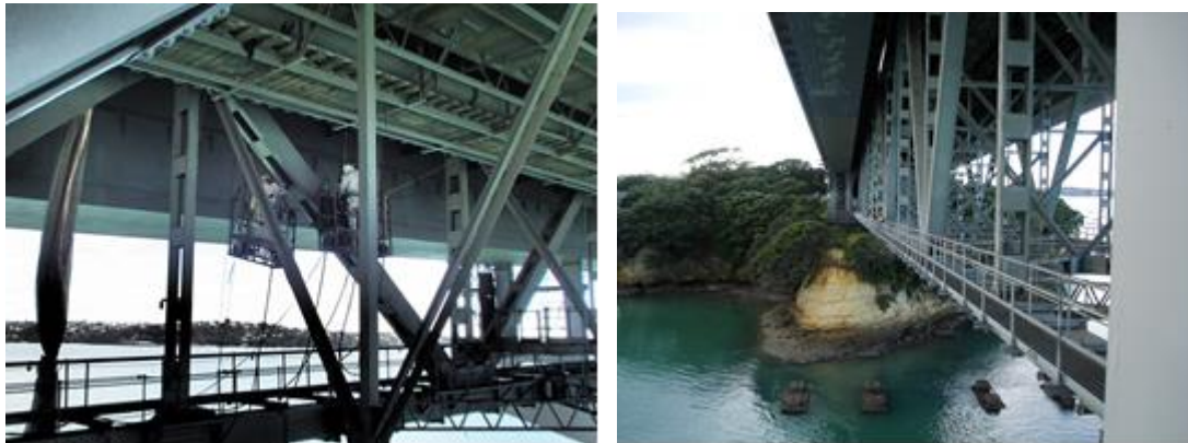
Figure 4: Typical spans over marine area requiring regular recoating maintenance
