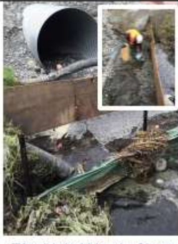
Silt fence, timber boards being used as a fish screen. Inset – Subcontractor salvaging silt from within the isolated work area.
