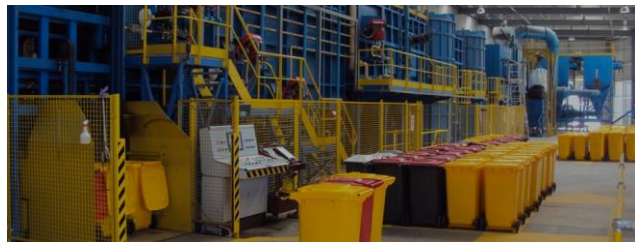
Thermal Destruction Plant (Hazardous and Bio-Hazardous Wastes) Dry Creek (2k tpa) - SA
